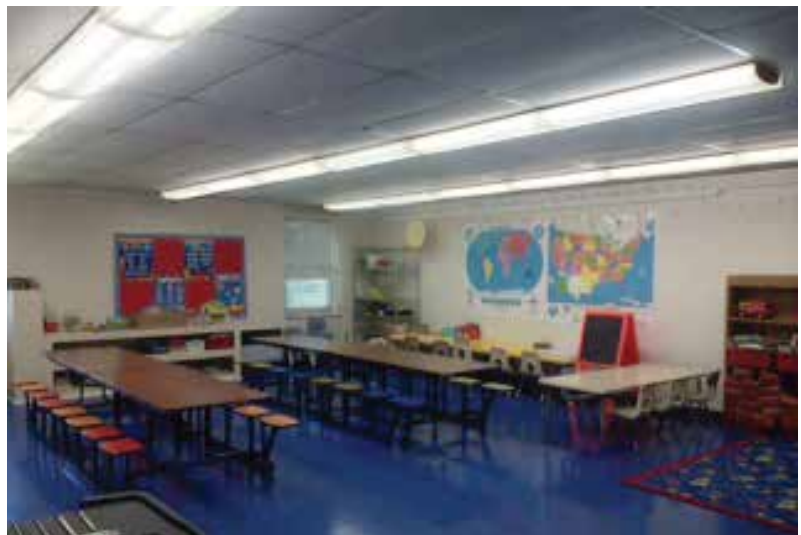
Class room change out by CRS Light. Replaced 40 watt magnetic ballasts with electronic ballasts. Replaced T12 fluorescent lamps with T8 LED Tube lights.
